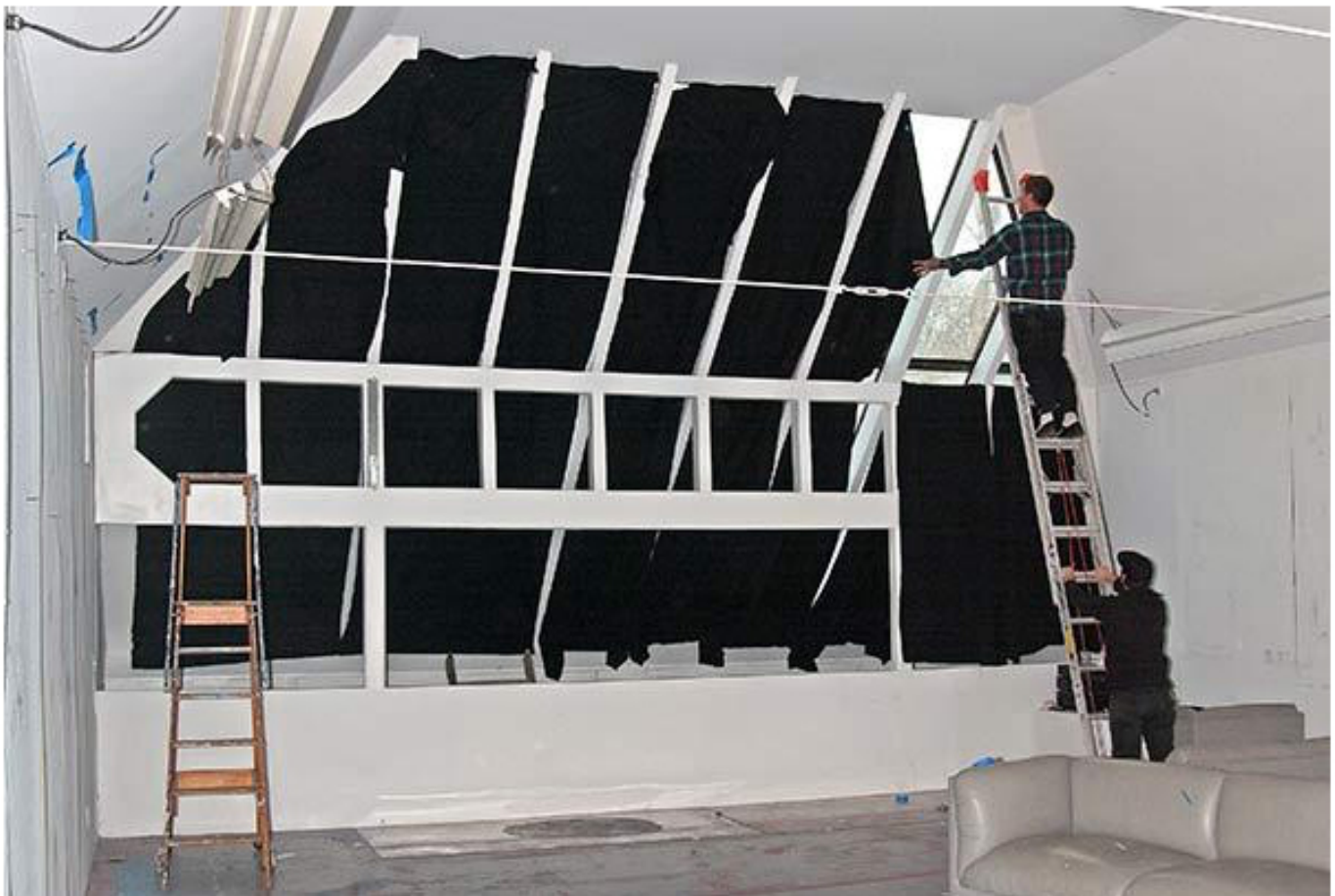
Chris Duncan installed black fabric over the windows of the de Kooning house in January 2014.
